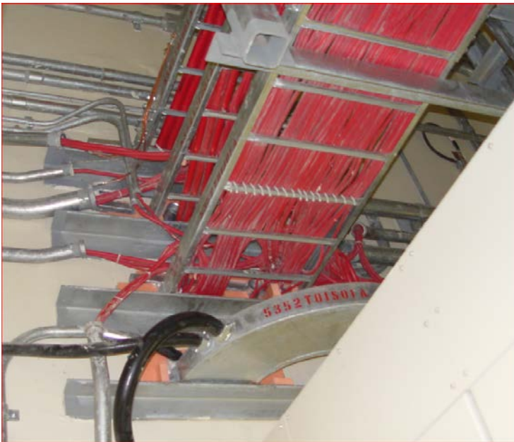
Figure 6.11.1. Example of interface between cable trays and conduits. Flexible conduits shall be used for Instrumentation and safety cables, being the aerial connection for non-safety power cables.
